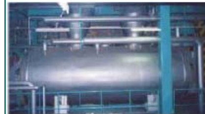
Tempura method facility
