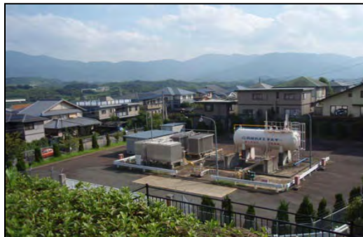
LP gas tanks
