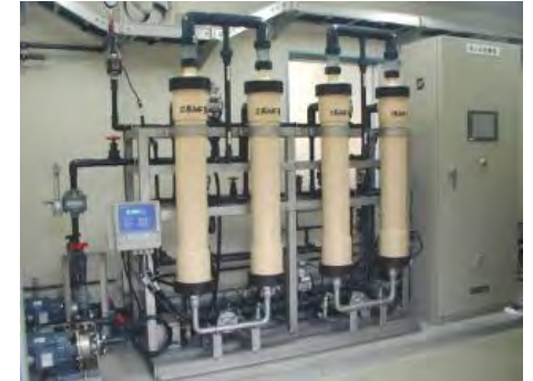
Membrane filtration system
