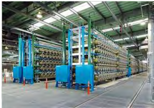
Sea water desalination system
