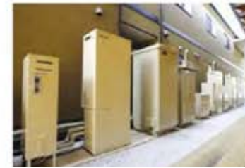
Fuel cell of the hydrogen demonstration house (Higashida H2)
