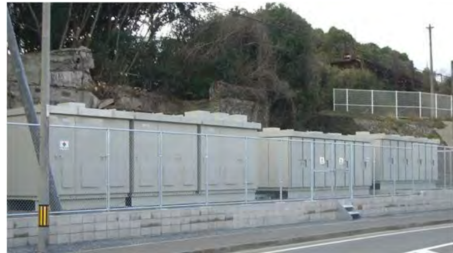
Large Capacity Secondary Battery (300kW) - Community Type
