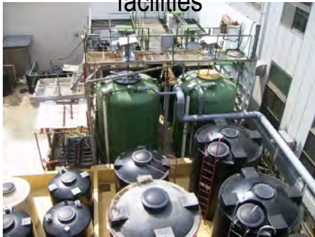
Neutralization • Storage facilities
