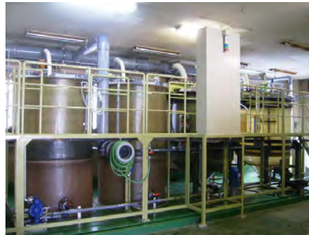
Oxidation* reduction facilities
