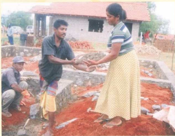
Hambantota resident Gunapala's daughter-in-law Ajantha helping construction workers at the site where the family's new home is coming up.
