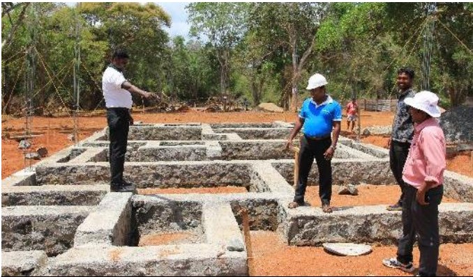
Construction of Teachers' Quarters at Periyakunchukulam Roman Catholic Tamil Mixed School is in progress.
