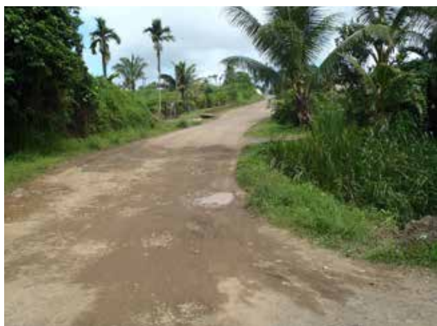
Poor road maintenance © SCOPE
