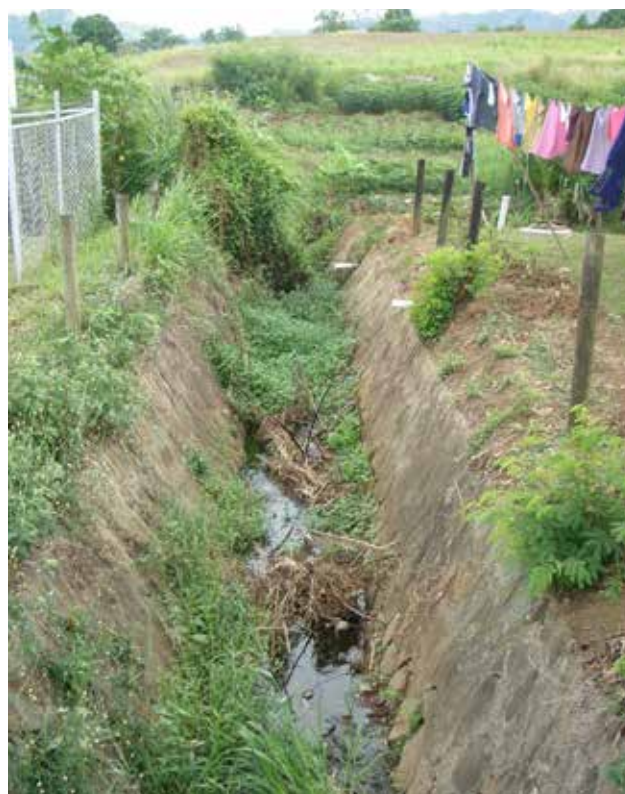
Poorly maintained drains in Nadi © SCOPE
