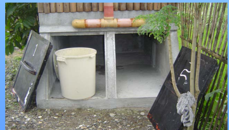
2-chambered vault: on-site treatment
