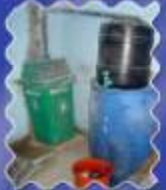
Urinal & Faucet collection tanks at the basement
