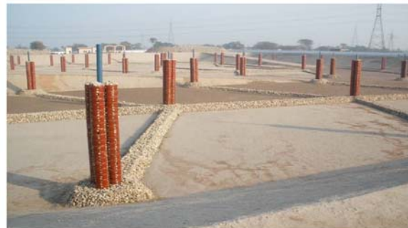
A VIEW OF TRENCH AT SANITARY LANDFILL SITE (LFS) AT MOUZA HABIBA SAYAL MULTAN.
